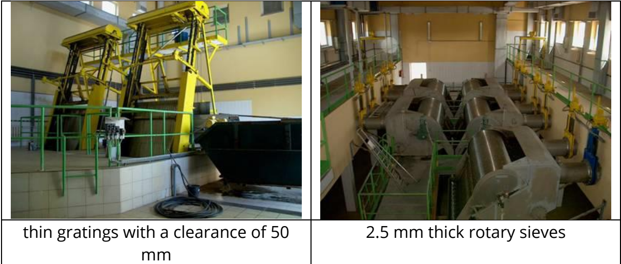
Photo.3 Screenings separation equipment ( www.zwik.zgora.pl )
